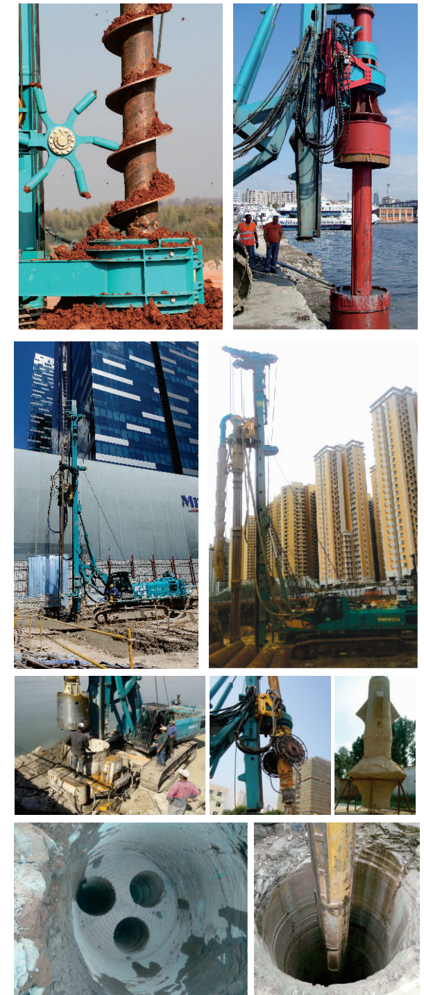
CFA, casing driven, High pressure jet grouting, large diameter DTH hammer, equipped with casing oscillator, DX Pile, drilling rock efficiently...
